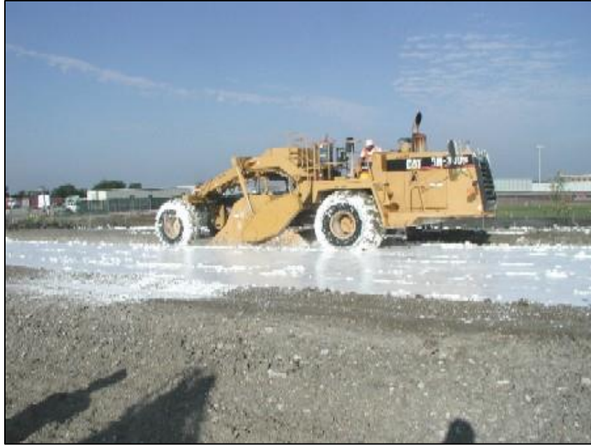
Photograph 19: Mixing a lime slurry into subgrade soils to reduce the swell potential.
