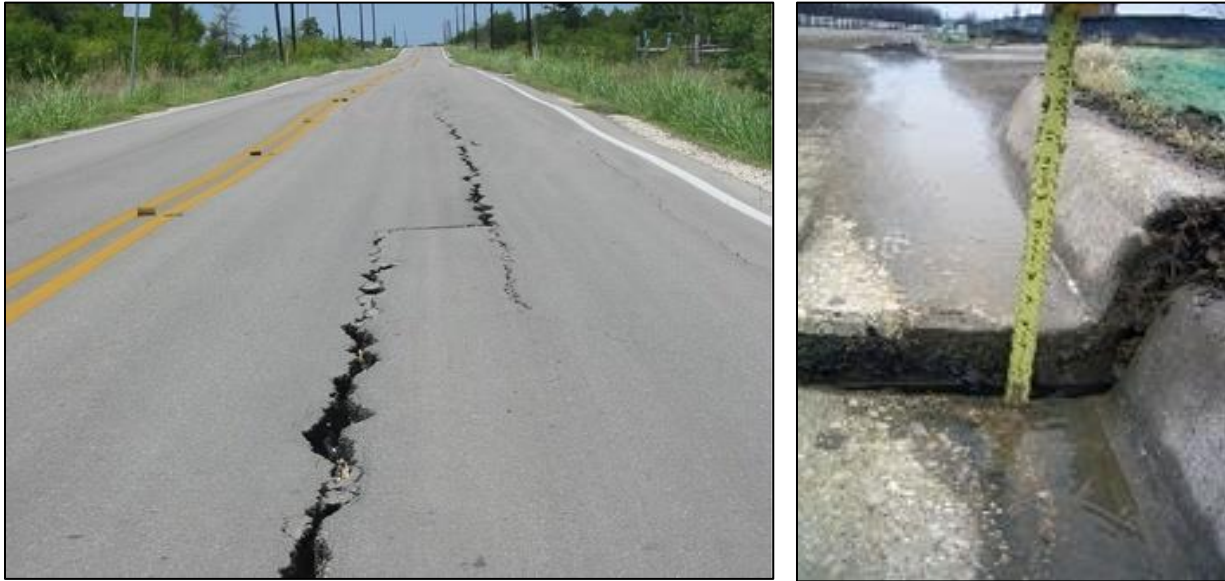
Photographs 17 and 18: Damage to asphalt pavement and separation along a concrete construction joint as a result of swelling soils.
