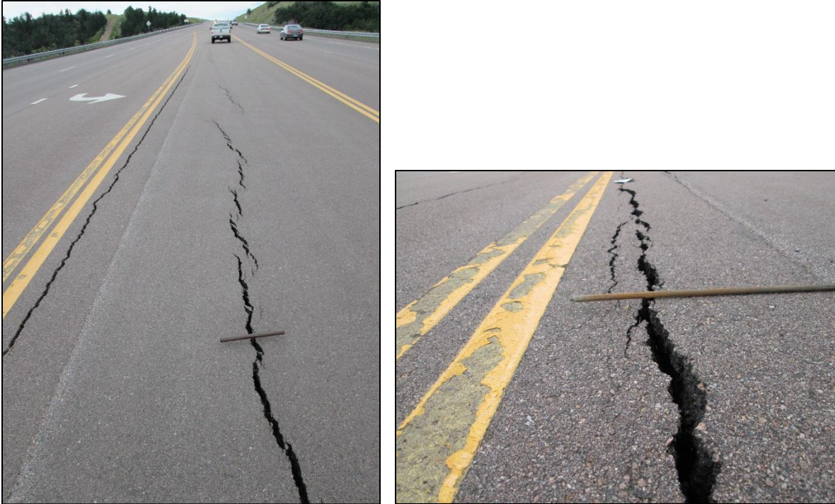
Photographs 11 and 12: Resultant pavement damage due to differential settlement caused by consolidation of saturated clays beneath a high embankment.
