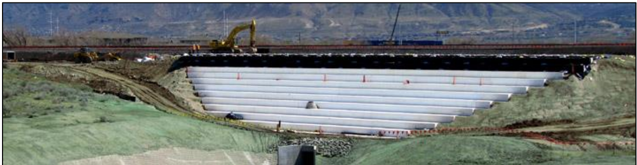
Photograph 15: Light-weight EPS foam blocks being used to bridge over soft clay deposits for new embankment construction.
