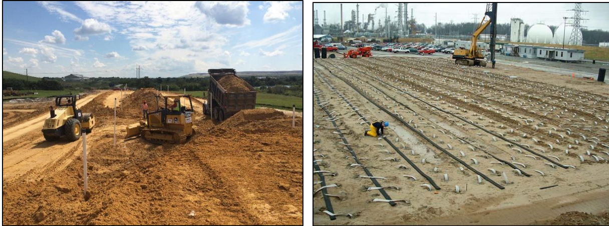
Photographs 13 and 14: Accelerated consolidation being achieved through the use of surcharging and wick drains.
