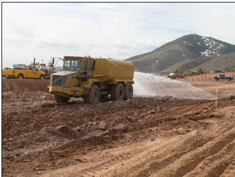
Photograph 6: Water truck being used to moisture condition soils in preparation for compaction.
