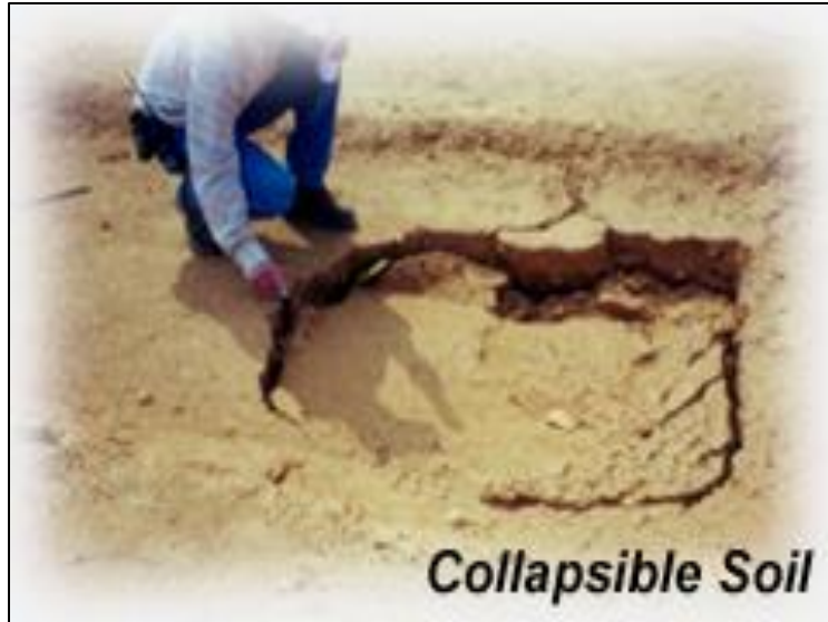
Photograph 20: Sinkhole development as a result of collapsible soil deposits settling at depth.
