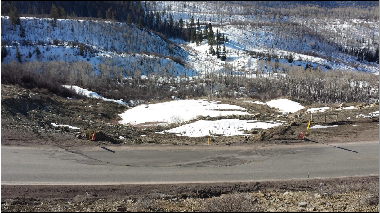
Photograph 16: Landslide that developed as a result of embankment construction over a weak clay deposit.
